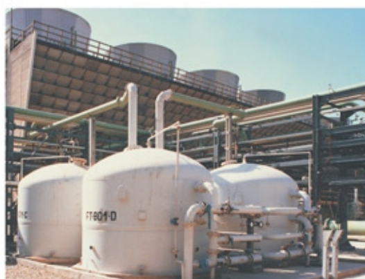
Cooling water treatment
