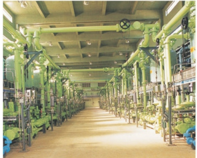
O & M services at power station
