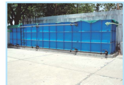
Fluidised Media Reactor in einem Hotel
