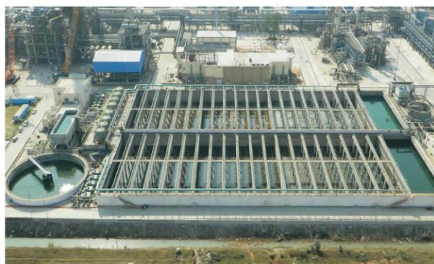
钢铁行业的污水处理厂
