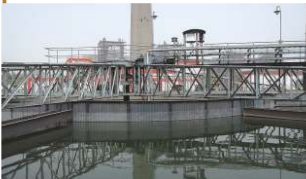
High rate solids contact clarifier
