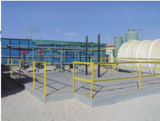
Packaged sewage treatment plant (200 m 3 /d fluidised media reactor) supplied to Gulf Petrochemicals Services & Trading (GPS) for the camp (1000 – 1200 people) located at Mukhaizna site where GPS was executing a project for Occidental Oman. The plant was delivered to site within three months and its erection and commissioning completed in 40 days
