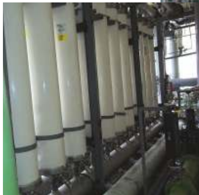
Ultra filtration stream
