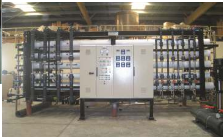
Four stream reverse osmosis plant of 3850 m 3 /day, supplied to Petroleum Development of Oman (PDO) at Faud site, Sultanate of Oman
