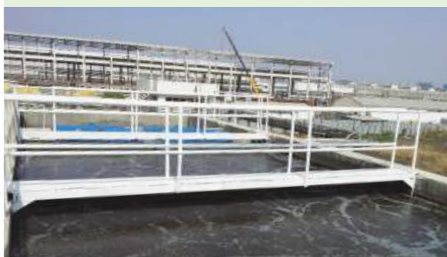
370 m 3 /d sewage treatment
