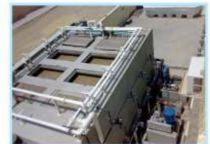
Membrane Bioreactor at Commercial Complex
