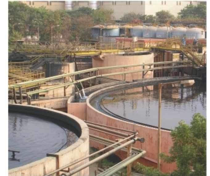
Management of complete water circuit at JSW Steel
