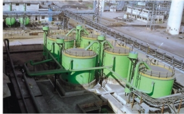
Part of water treatment system supplied to Bhushan Steel and Strips Limited
