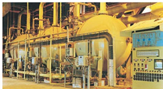
Condensate polishing units
