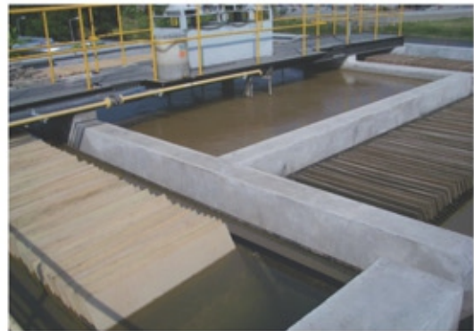
Ultra high rate clarifier
