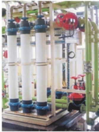
Ultra filtration plant
