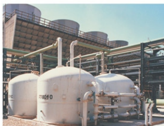
Cooling water treatment
