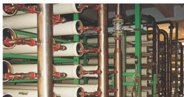
Zero discharge plant
