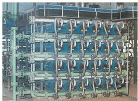
Sea water reverse osmosis desalination plant
