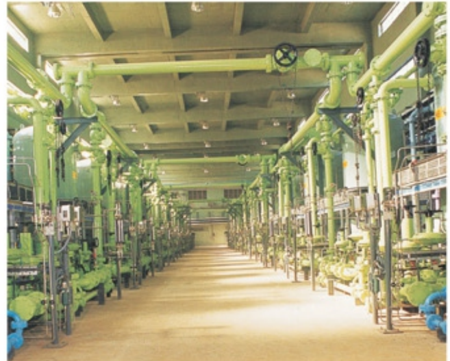
O & M services at power station
