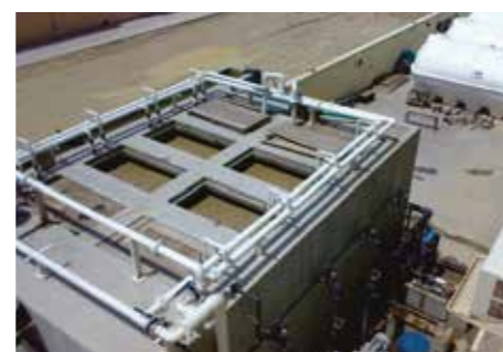
INDION Membrane Bio-reactor (MBR)
