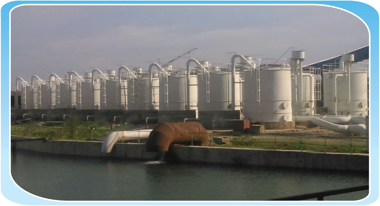
18 units comprising 160 m 3 /h capacity at BHEL, Uttar Pradesh
