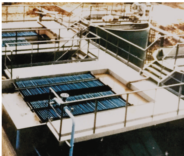
Installation in India of 2 x 100% Lamella Clarifiers with flocculation tanks. Each clarifier is rated for a maximum flow of 240 m 3 /h
