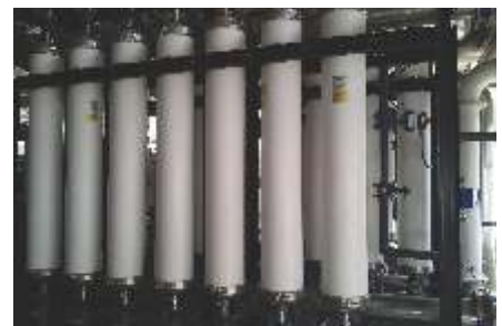
Ultra Filtration Plant
