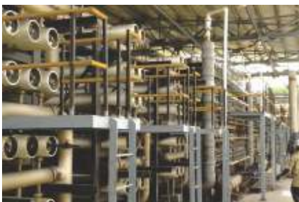
Reverse Osmosis Plant
