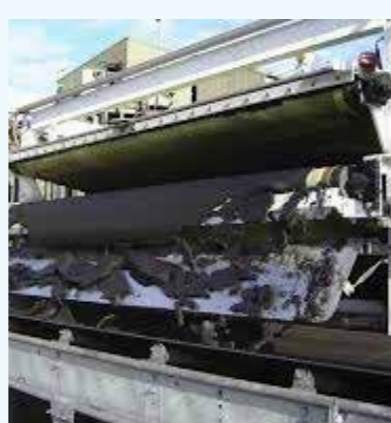
Belt Press for Coal Slurry
